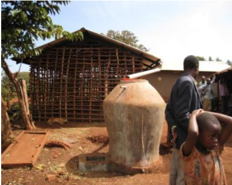
Figure 4.4 DRWH Jar Constructed by NGO in Kapchorwa District
