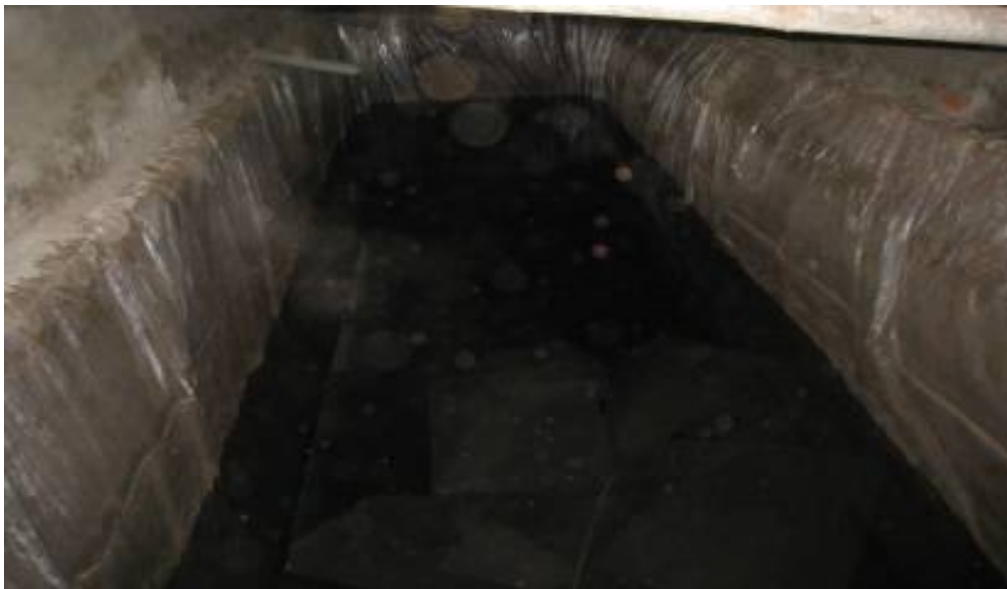
Figure 4.7 Commercial Rainwater Harvesting Facility in Kigangazi Trading Centre, Masaka District
