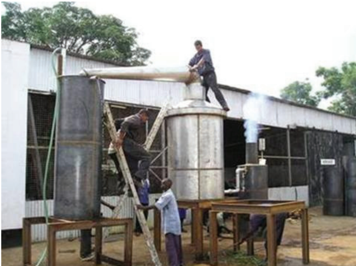
Figure 5. Technicians undertaking a trial run of the newly constructed essential oil distillery.
